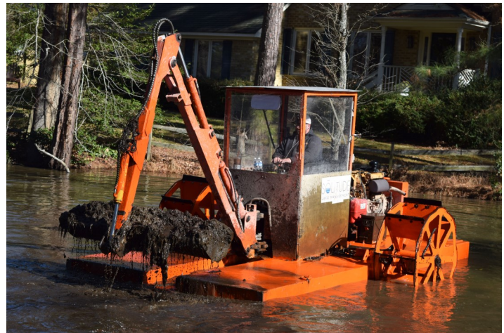
Hydro-raking can be an extremely effective management tool for the removal and reduction of nuisance aquatic plants found in community lakes, stormwater ponds and private waterbodies.
