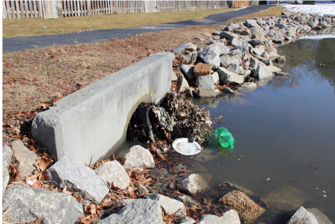
Clogged Inflow Pipe
