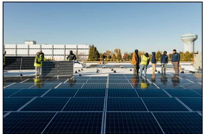
Photo credit: Julian Bracero / EmPower Solar - The Grumman Community Solar Project
