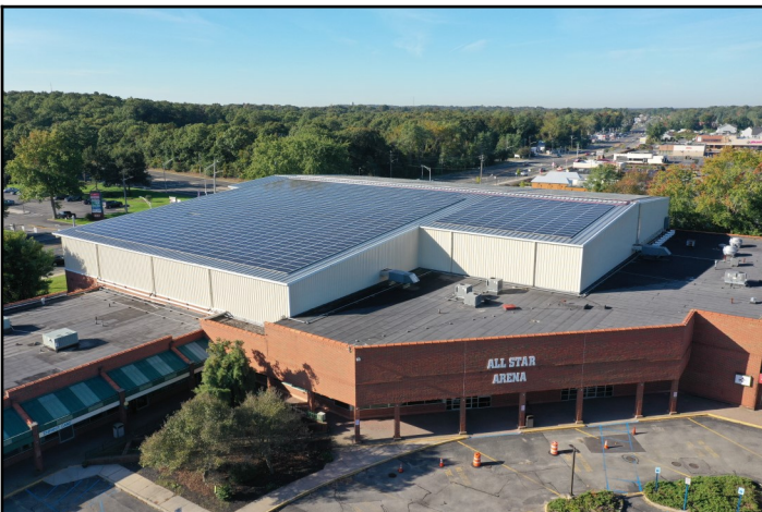
Photo credit: Anthony Pasini / EmPower Solar - The Selden Community Solar Project
